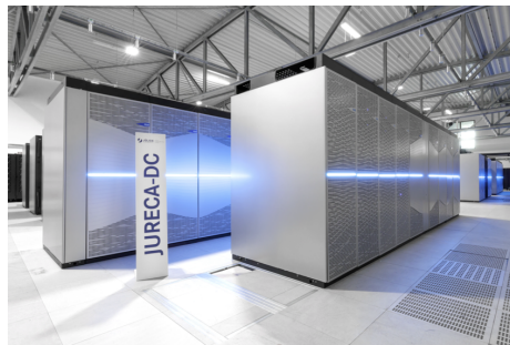
Figure 2.16: The JURECA-DC module at Jülich Supercomputing Centre. Image taken from [Figure 1][152] under CC BY 4.0 licence. Copyright: Forschungszentrum Jülich GmbH / Ralf-Uwe Limbach.
