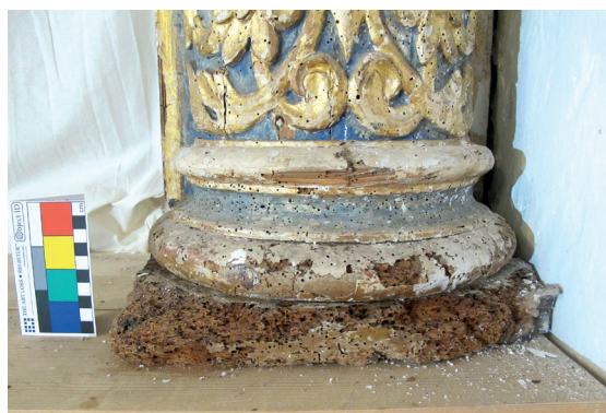
Fig. 167: St Mary retable, plinth of the right column, condition as found; deterioration of wood
