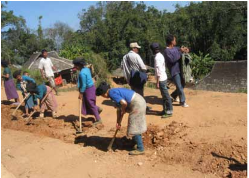
Trench Digging for water supply distribution system in Nar Wai Village, Wa special Region, Myanmar
