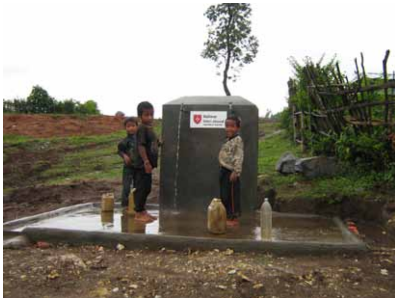
Gravity Flow water system Lai Rai, Wa Region, Myanmar
