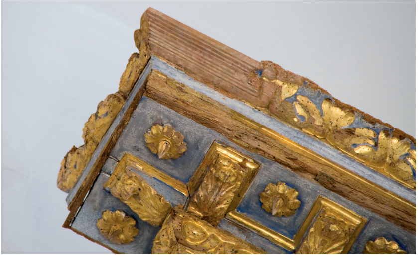
Fig.36: Right gable; reconstruction of the broken corner
