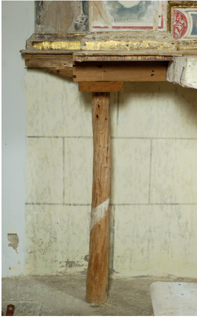
Fig. 75: Painted square pattern of masonry joints became visible after the removal of the modern paneling of the pedestal zone
