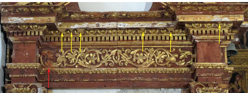
Fig. 170: St Joseph retable, condition as found; clearly visible losses in gilding, the upper contour of the entablature is destroyed by insects. Many of the separately carved diamond-shaped applications are lost. Yellow arrows indicate the few surviving ones. The red arrow indicates the area where the gilding shows a reddish discoloration.
