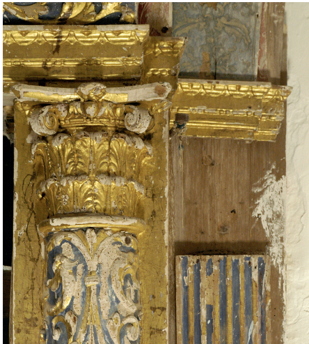
Fig. 104: Upper part of left column and pilaster; condition as found, the capital of the pilaster is missing
