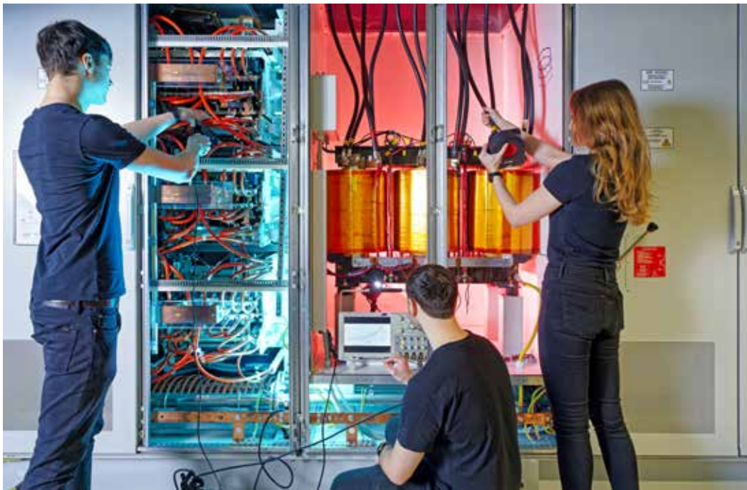
Figure 8.5 E.ON ERC|PGS assistants preparing a 5 MW DAB for testing. A 5.0 MVA, 1,000 Hz dry-type transformer is used for galvanic isolation. With a total weight of 675 kg, 0.140 kg per kVA is needed (with permission).
