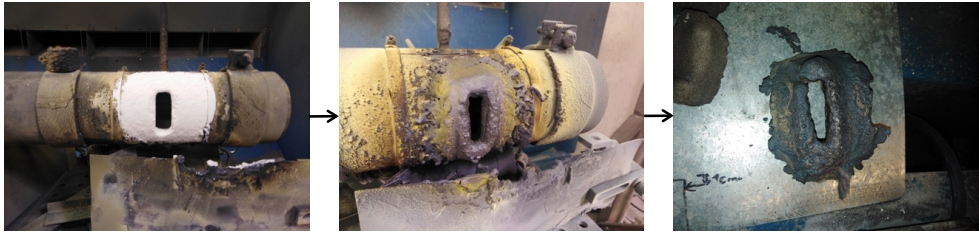
Figure C.3 Clogging of the slit at the shrouding chamber, which needs to be manually removed
