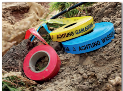
Figure 16: pipe warning tape
