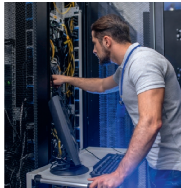
DATA DRIVEN: Tech organizations need more server capacity to keep up with demand.
