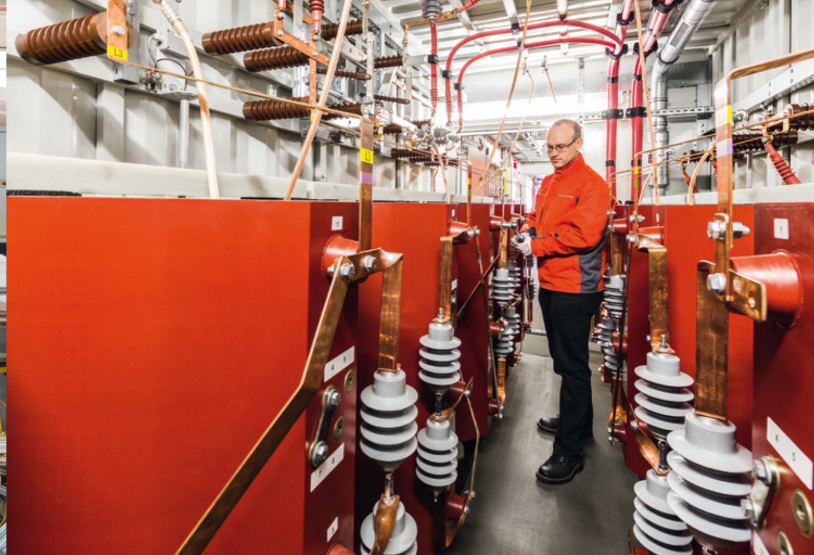
Low-Voltage Ride-Through (LVRT) Container
