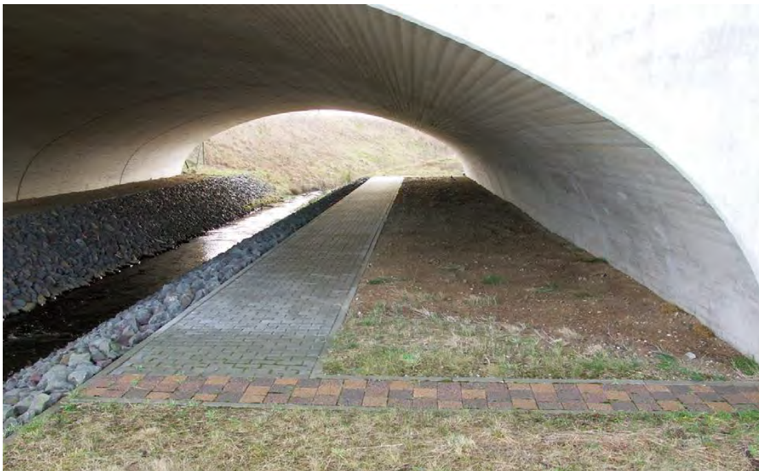
Fig. 23: Poor design of water course passages
