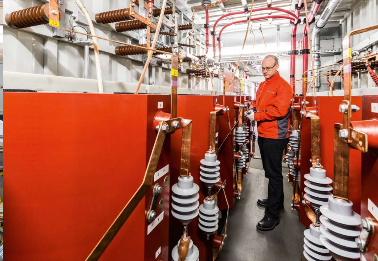
Low-Voltage Ride-Through (LVRT) Container
