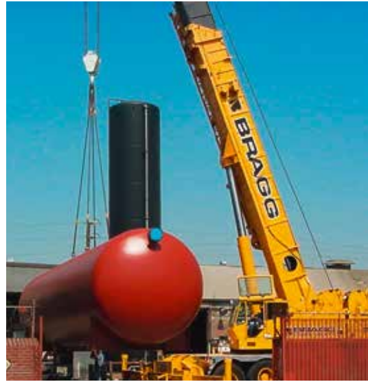
Large-scale thermal storage tank
