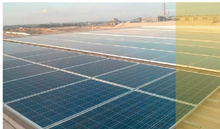
Image 3: PV Installation carried out by Spectra - Energies Renouvelables at Sfax (Source: Spectra)
