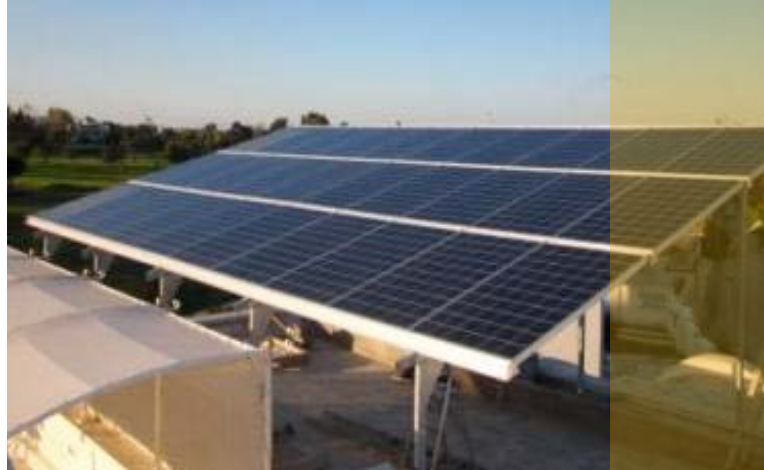
Image 2: PV installation carried out by WS.Energy (Source: WS.Energy)
